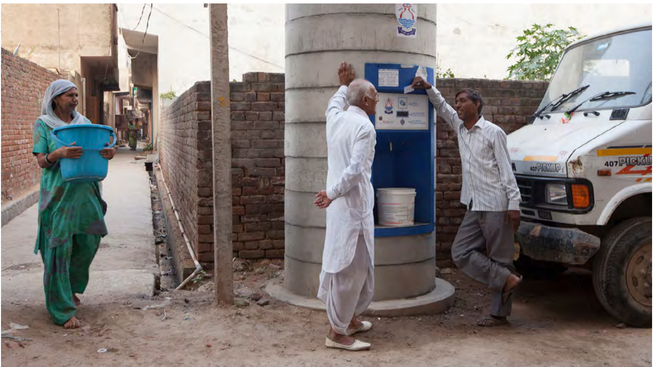
The solar powered vending machines installed by a for-profit social enterprise called Piramal dispense clean drinking water via a pre-paid smartcard to residents who have no access to water on tap in their homes. New Delhi, India. (Photo by In Pictures Ltd./Corbis via Getty Images)
